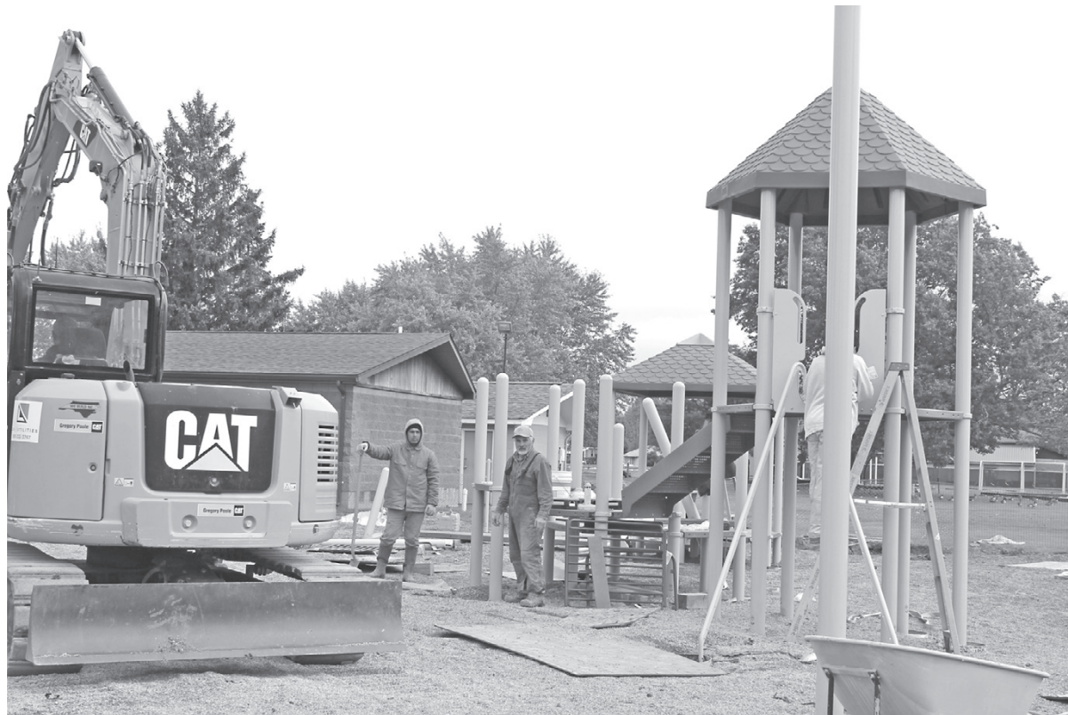
Workers with Gardenville Landscaping of West Seneca assemble the components of the inclusive playground being built in Fairmount Park, Wheatfield.
